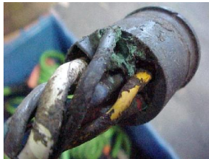
De-icing chemicals may find their way into plugs and sockets, causing irreversible damage
